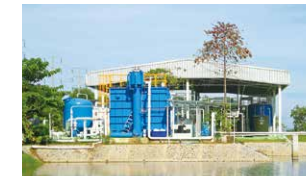
Rainwater basin and rainwater recycling equipment at the Bang Pa-in Plant in Thailand
